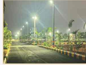
Electric Lines with Street Lights
